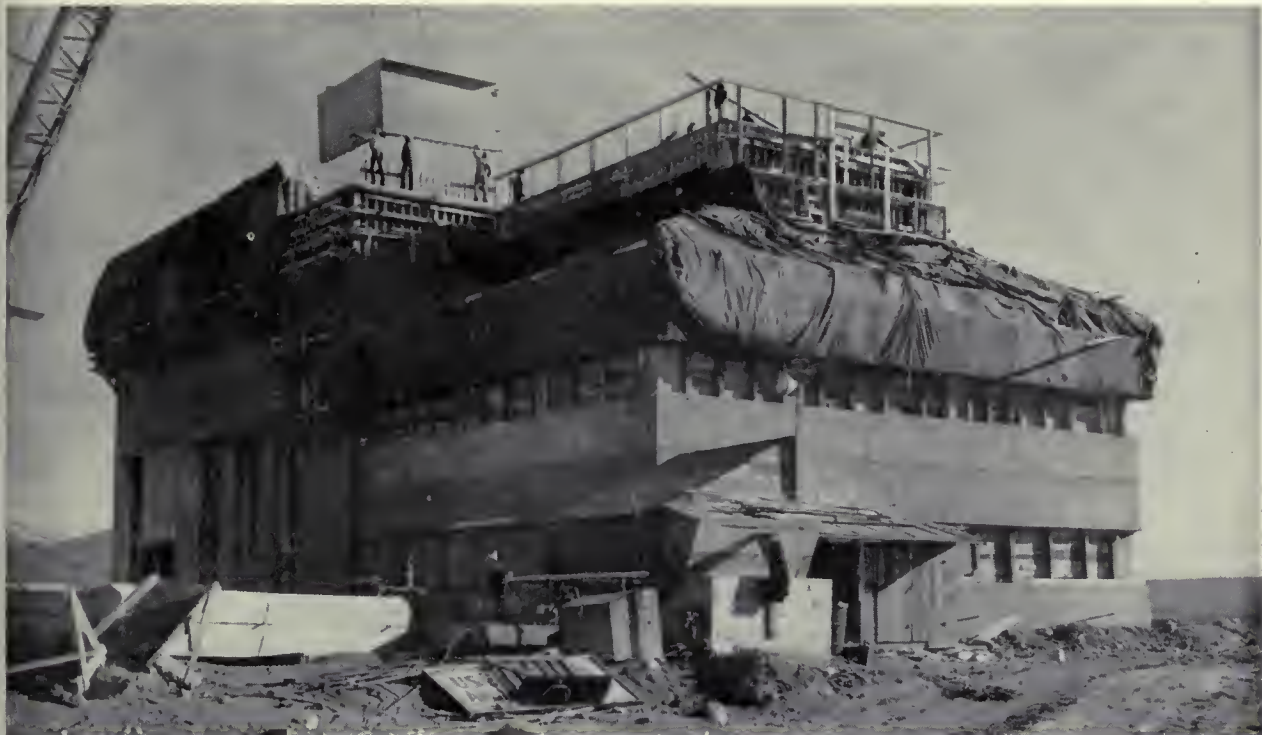
GRANBY PUMPING PLANT, the "mainspring" of the Colorado-Big Thompson project, as it appeared 2 years ago this September.
